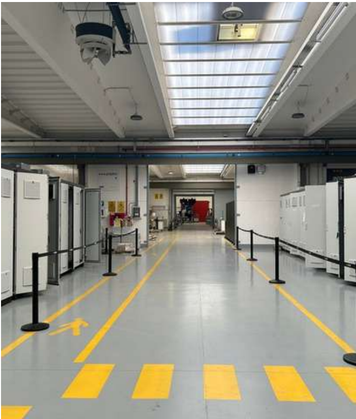
ELECTRICAL EQUIPMENT WORKSHOP
