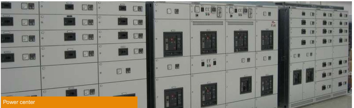
Turnkey electrical room in container
